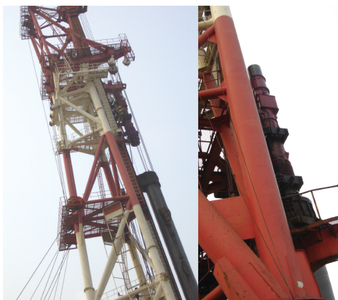
浙江杭州湾跨海大桥D180柴油锤 Hangzhou Bay Bridge, Zhe jiang. With D180
