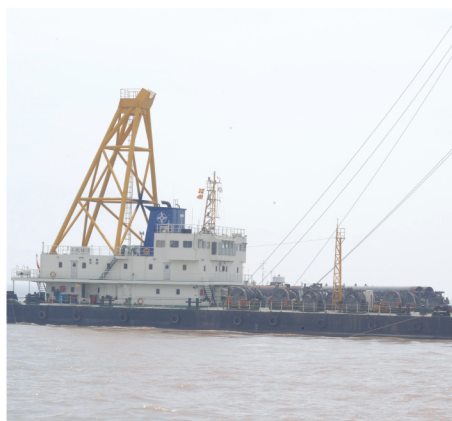
东海风电一期二期D220柴油锤 Donghai Bridge Wind farm, Shanghai. With D220
