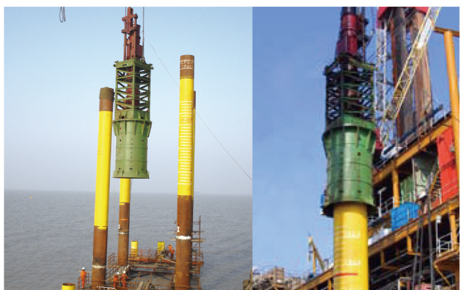
天津渤海湾石油平台D220柴油锤 Bohai Bay Offshore platform, Tianjing. With D220
